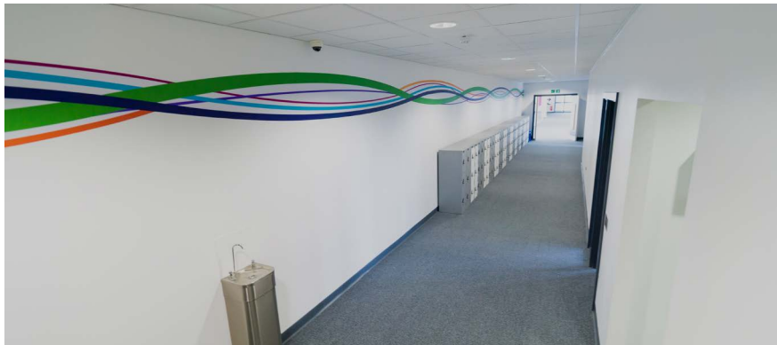
3 Circulation spaces lack daylight
